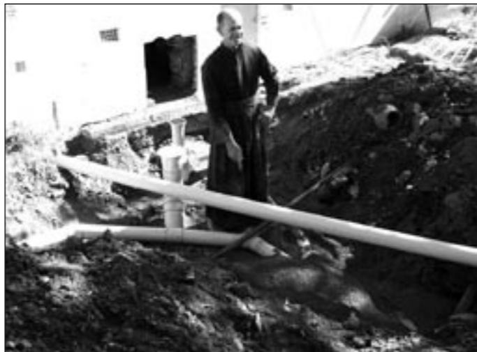
Bro. Joseph smiles over the new sewage lines before they are buried.
