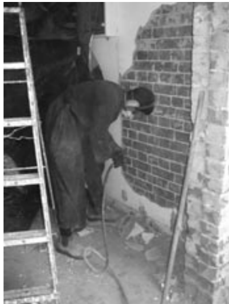
Bro. Francis removing the crumbling rendering from a wall damaged by moisture.
