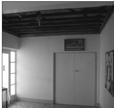
A view of the ceiling needing replacement after the plumbing work.
