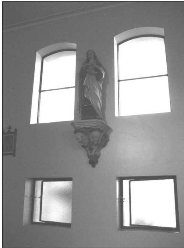
Some of the old single pane windows in the chapel that we hope to replace with more efficient windows, which hold the heat in during the winter and allow the air to flow in the summer.
