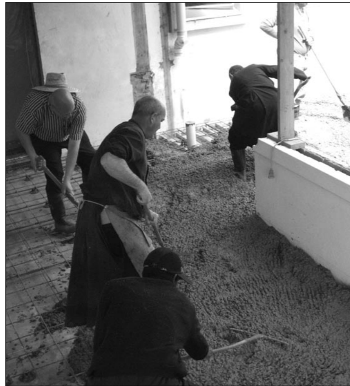
Concrete work on the Chapel Entrance for the faithful begins with the Brothers hard labour.
