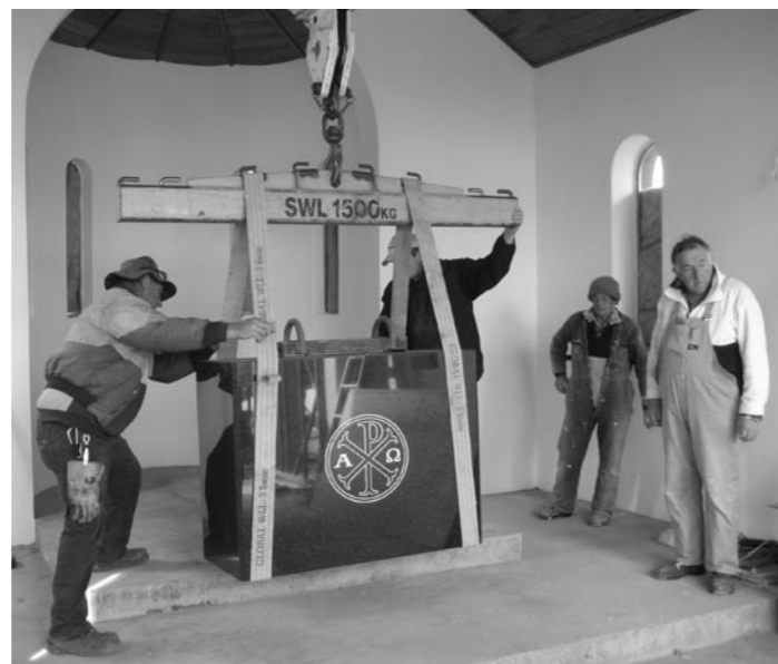
Work continues on the Seminary Cemetery chapel as the solid black granite altar is hoisted in place by crane. The altar has been installed and the remaining work to lay down the floor, complete the electrical work and painting awaits the help of our benefactors kind support. Please help us finish this work before the Feast of All Souls. Thank you for your support.
